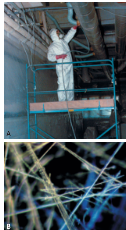
Fig. 2.17 Asbestos insulation is common in buildings and presents a hazard when disturbed during demolition. (A) Protective clothing must be worn to avoid contact with (B) asbestos fibres .
